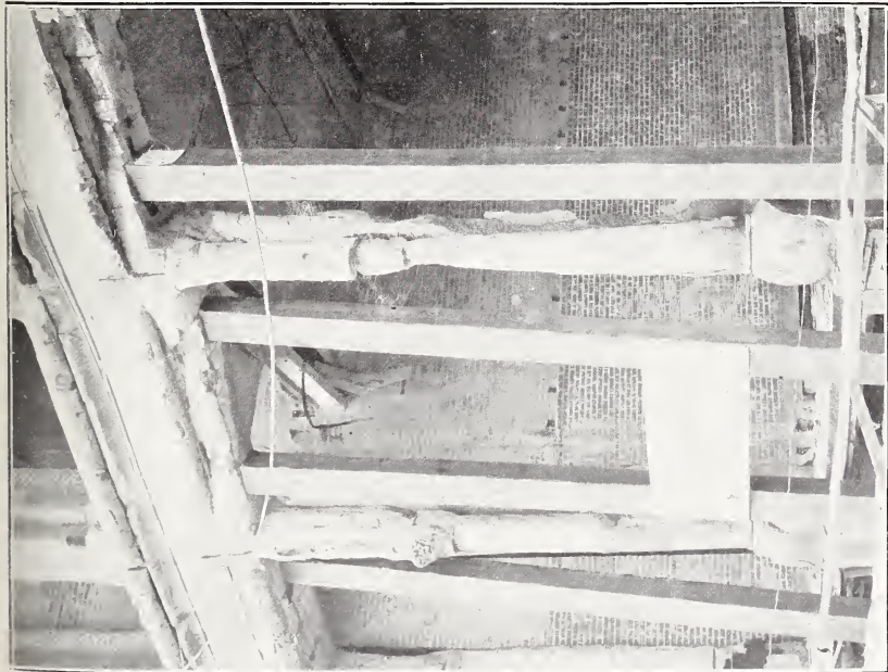
1. GRANITE COLUMNS SPALLED BY FIRE, HOBART BUILDING, SAN FRANCISCO.
